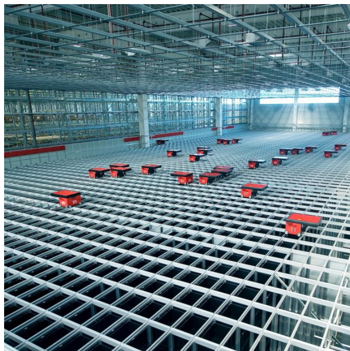
Figure 4.8: ©Autostore AS. Illustration of a physical installation of an Autostore System. The red taxi agents gather items from the bins in the grid and deliver them to delivery points.
